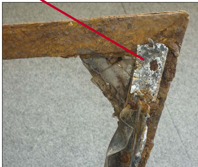
Inside view of the forward / top corner of the left window. The arrow is pointing to a metal plate, which overlapped the Perspex from the outside, surrounded by tube frame of the canopy.
